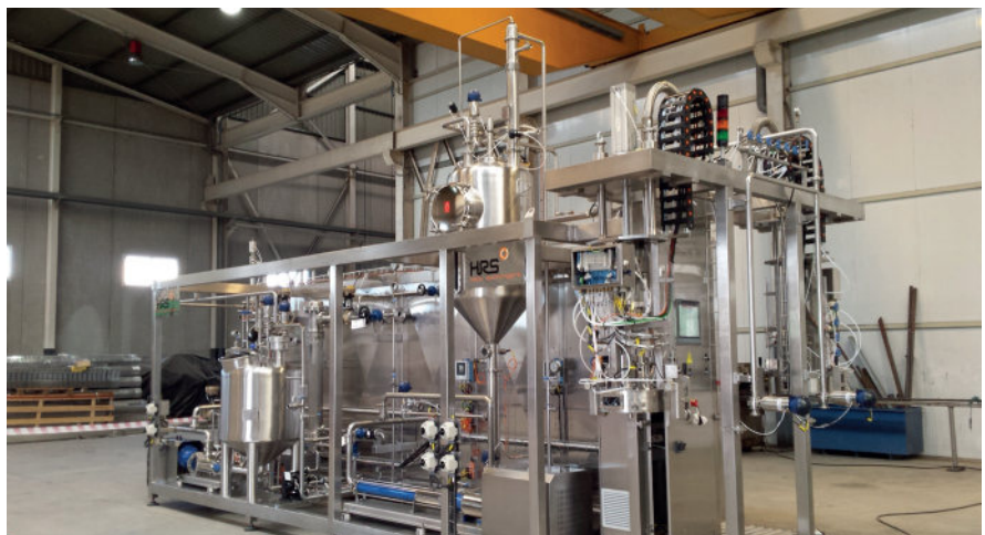
Control box installed to allow the reading from a monitor (such as a Brix meter) to control product recovery from an HRS heat exchanger.
