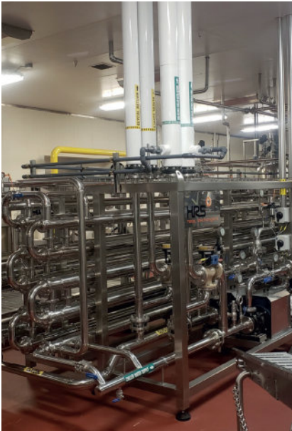
Part of the cooling system of a continuous system installed at a soup and sauce manufacturer
